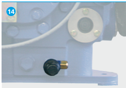
Oil service valve
