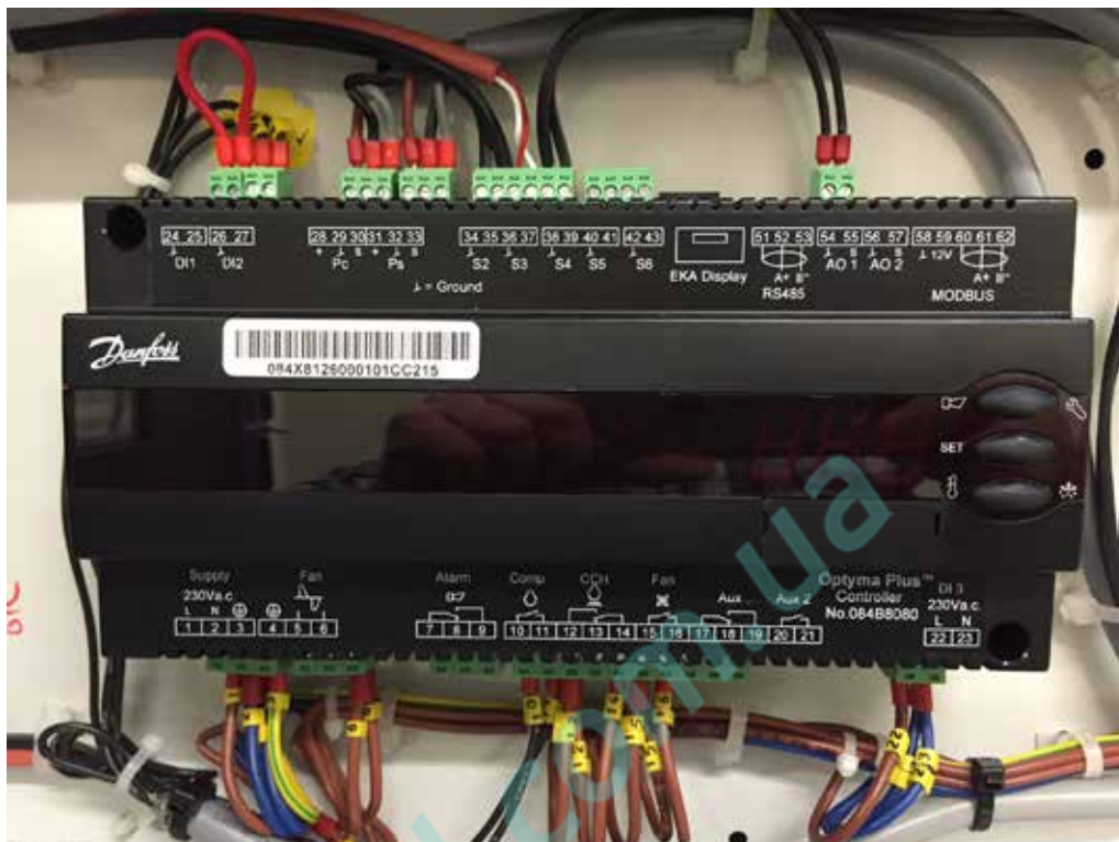
Picture1. Normal wiring
