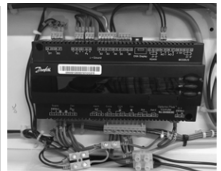
Picture 4 : Temporary wiring
