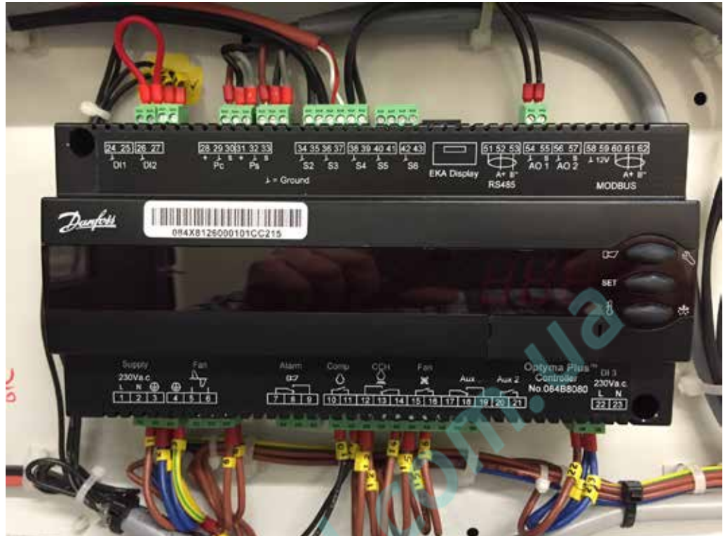
Picture1. Normal wiring
